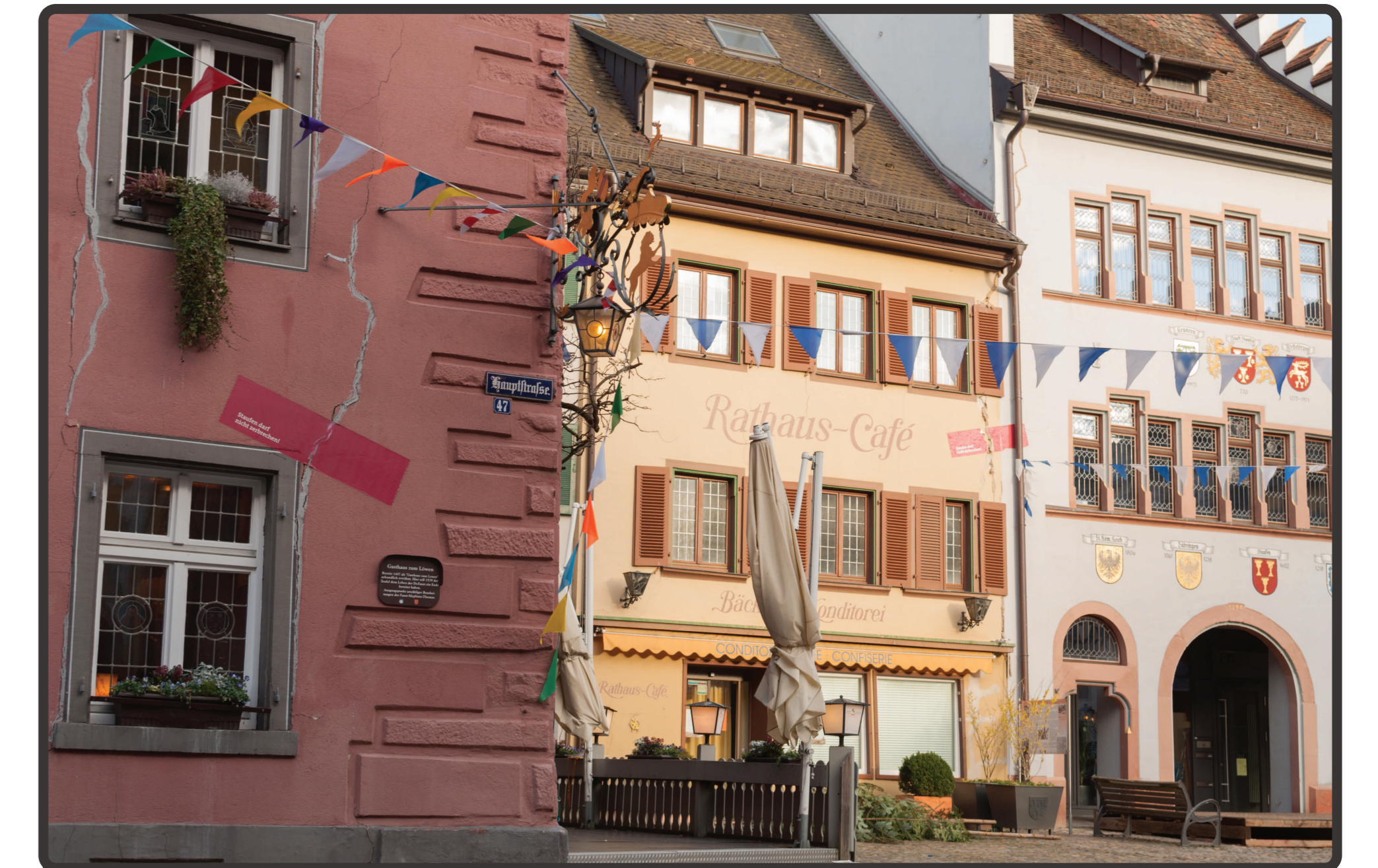
Staufen im Breisgrau, damaged houses as a result of ground heave after thermal drillings.
