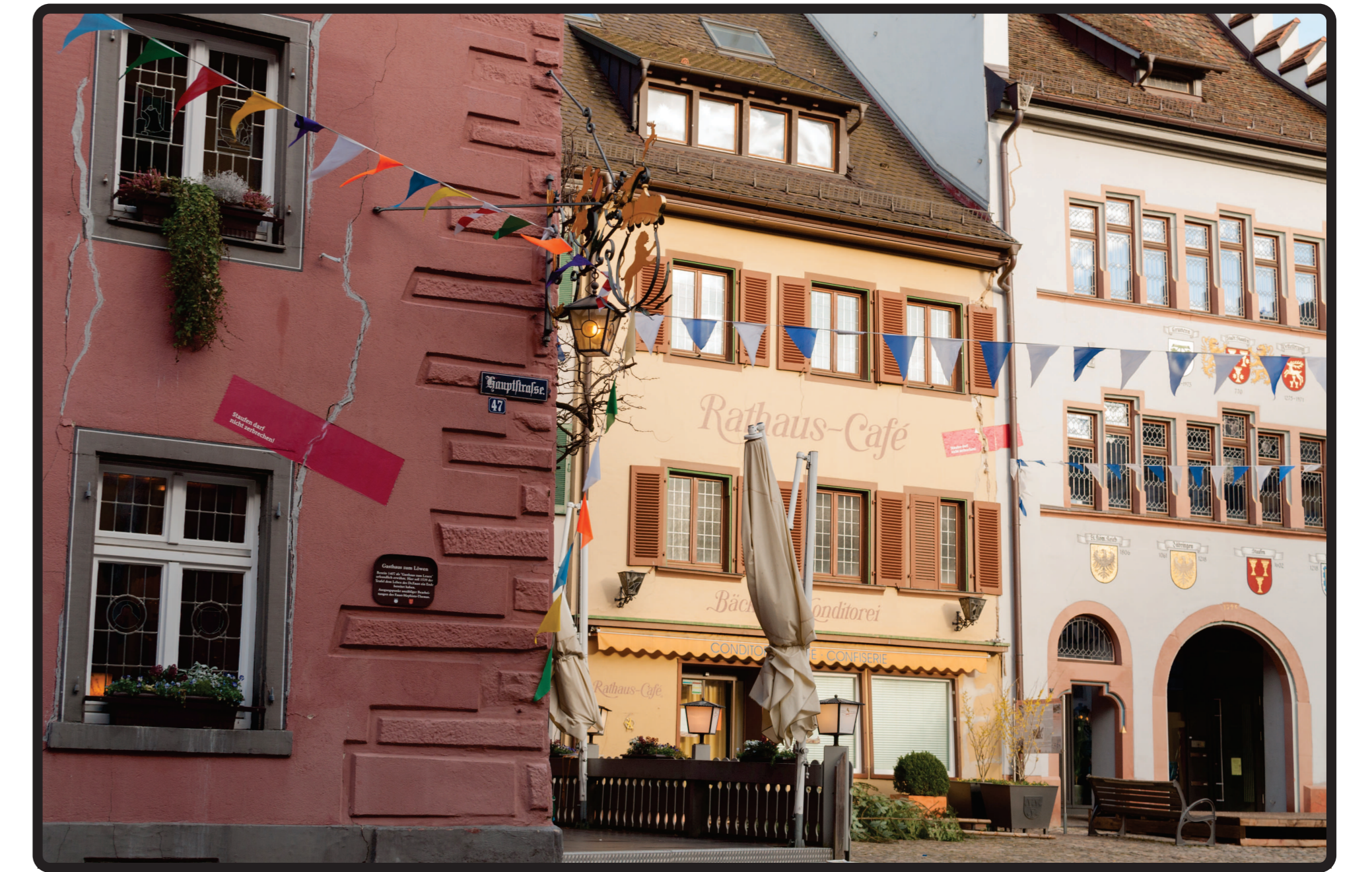
Staufen im Breisgau, damaged houses as a result of ground heave after thermal drillings.
